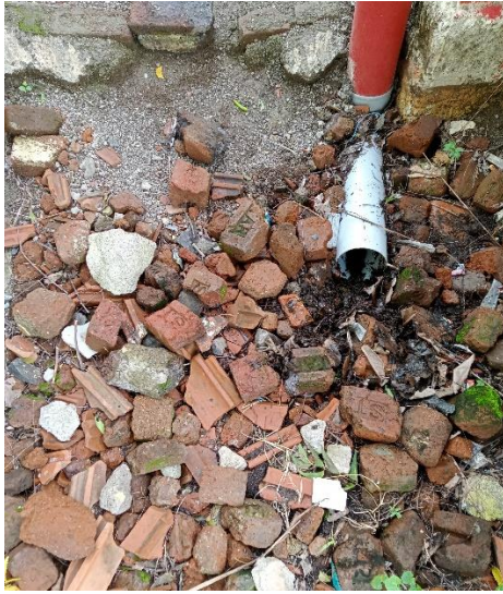
RAIN WATER HARVESTING PIT
