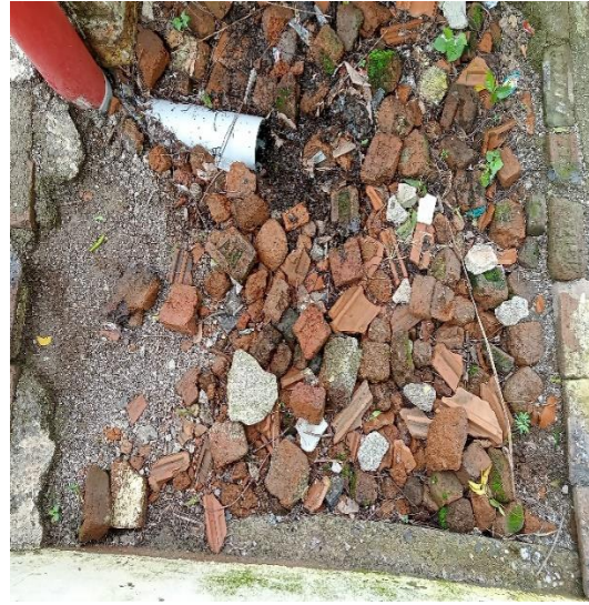
RAIN WATER HARVESTING PIT
