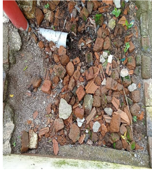
RAIN WATER HARVESTING PIT
