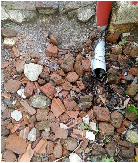
RAIN WATER HARVESTING PIT
